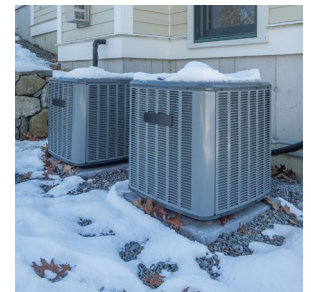
Air Conditioning Units
