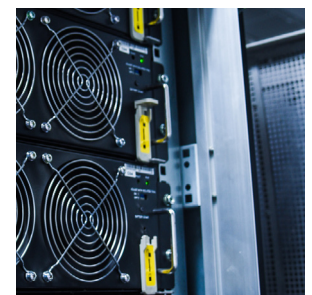
Data Storage Equipment
